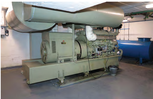
Cold War generator at Steintorwall Bunker which remains in excellent condition
